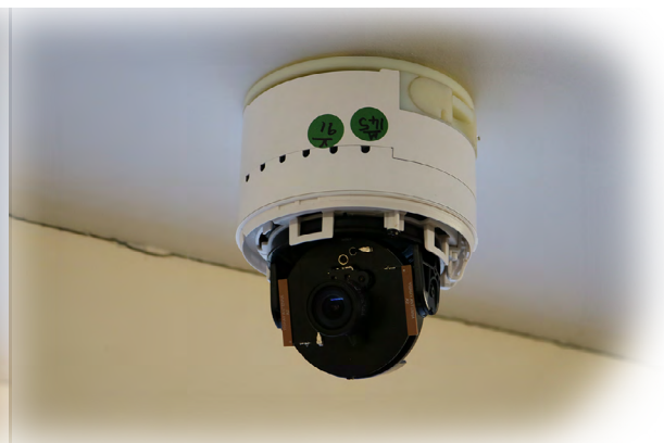
Black plastic dome removed
